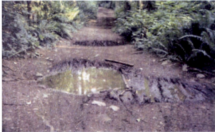
Photo 8. Degradation of an unsanctioned trail by overuse in wet conditions (Anon.).
